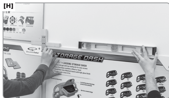
H] ** 2-PERSON JOB** Using the Install Jig on the right edge, position the next Bottom Panel, make sure it's level, and then mark all 4 mounting locations.
